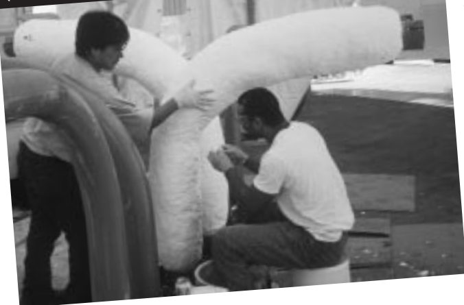
Technicians apply "pack in place" insulation to Pipeline End Manifolds (PLEMS) for the Shell King project.
